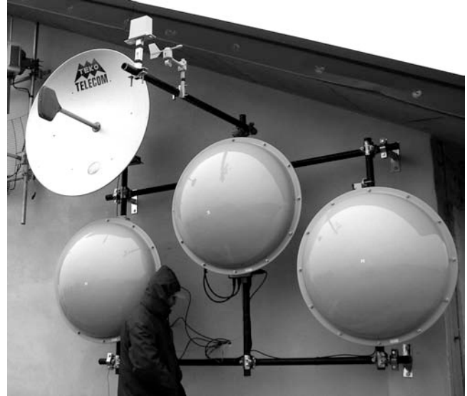
Figure 5: Physical installation at Monte Cesen.
